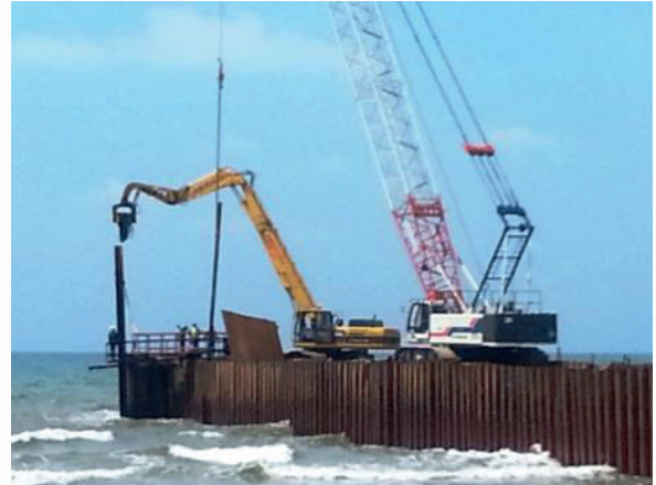
Cofferdam sheet piling works using combination of Crawler Crane and excavator mounted vibro hammer
