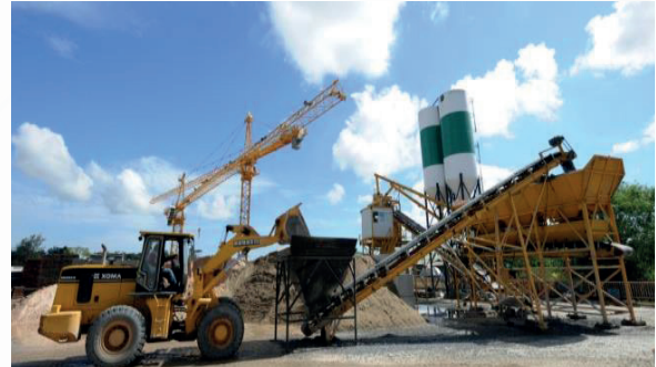
In-house computerised wet-mix batching plant
