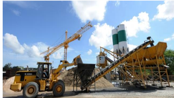
In-house computerised wet-mix batching plant
